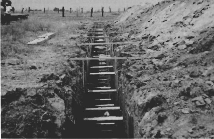
Figure 1. A typical backhoe trench excavated across the active San Jacinto fault zone.
